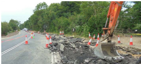
The old pavement to the side of the new road is being dug up. This will be laid as a verge with planting to the approach to the new roundabout
