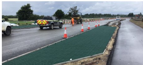
Construction of the maintenance lay-bys which provide stopping opportunities for road users needing to stop for a short duration
