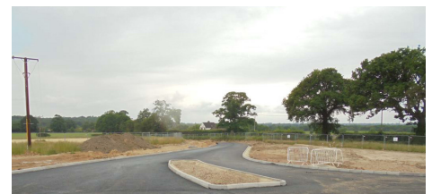
New asphalt laid around the Swallowfield Road arm of the new staggered junction
