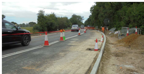
New carriageway kerb lines laid at western tie-in with Bridge Farm roundabout
