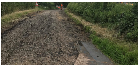
Works are progressing along section of Swallowfield Road between junction with Greensward Lane and Castle Hill
